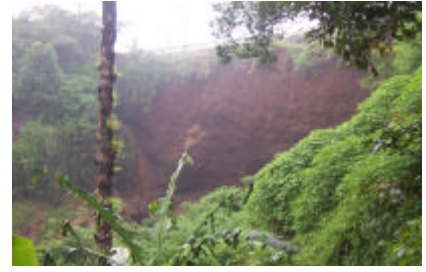
Cipanas Failure, March 10 th 2005
